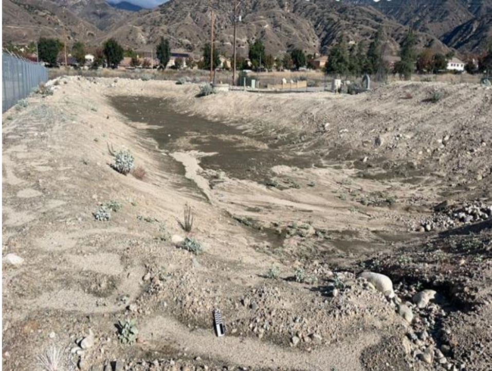
Figure 5. General View of Depression of the Discharged Pipeline on the Northwest Section of the APE, View NW
