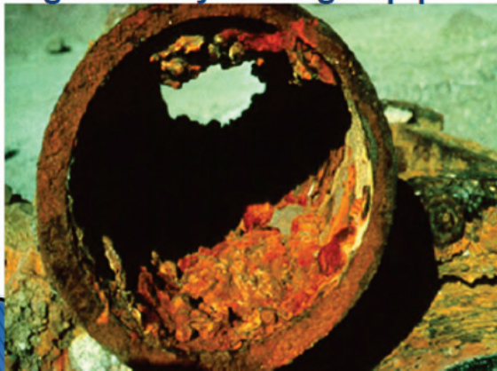
High salinity damages pipes
