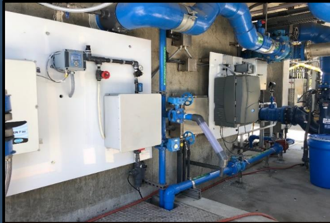
On-line Instruments Installed
