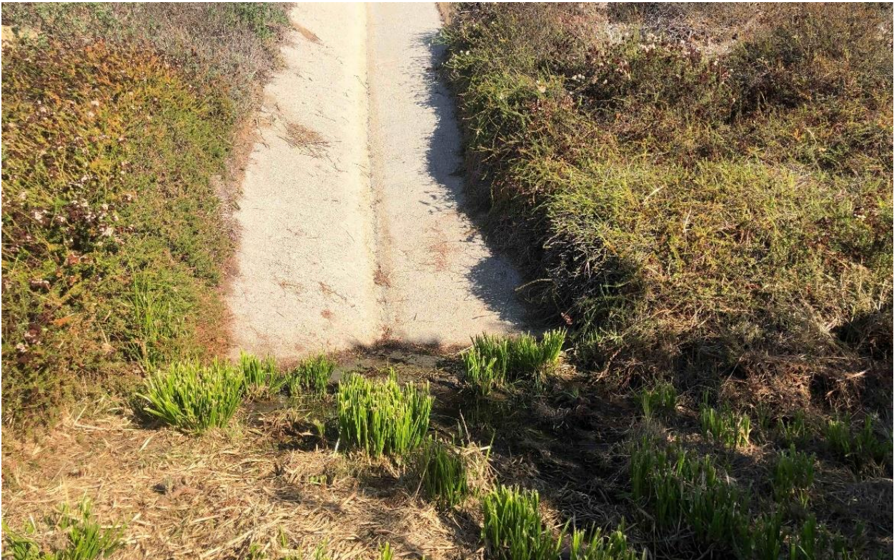
Photograph 2. Surface water seeping from beneath v-ditch into Basin 1, facing northeast.
