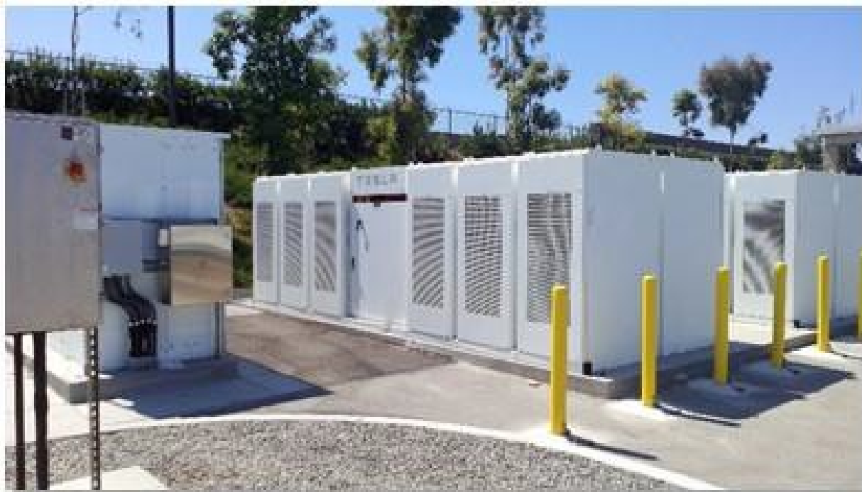
Figure 9 Example BESS Facility
