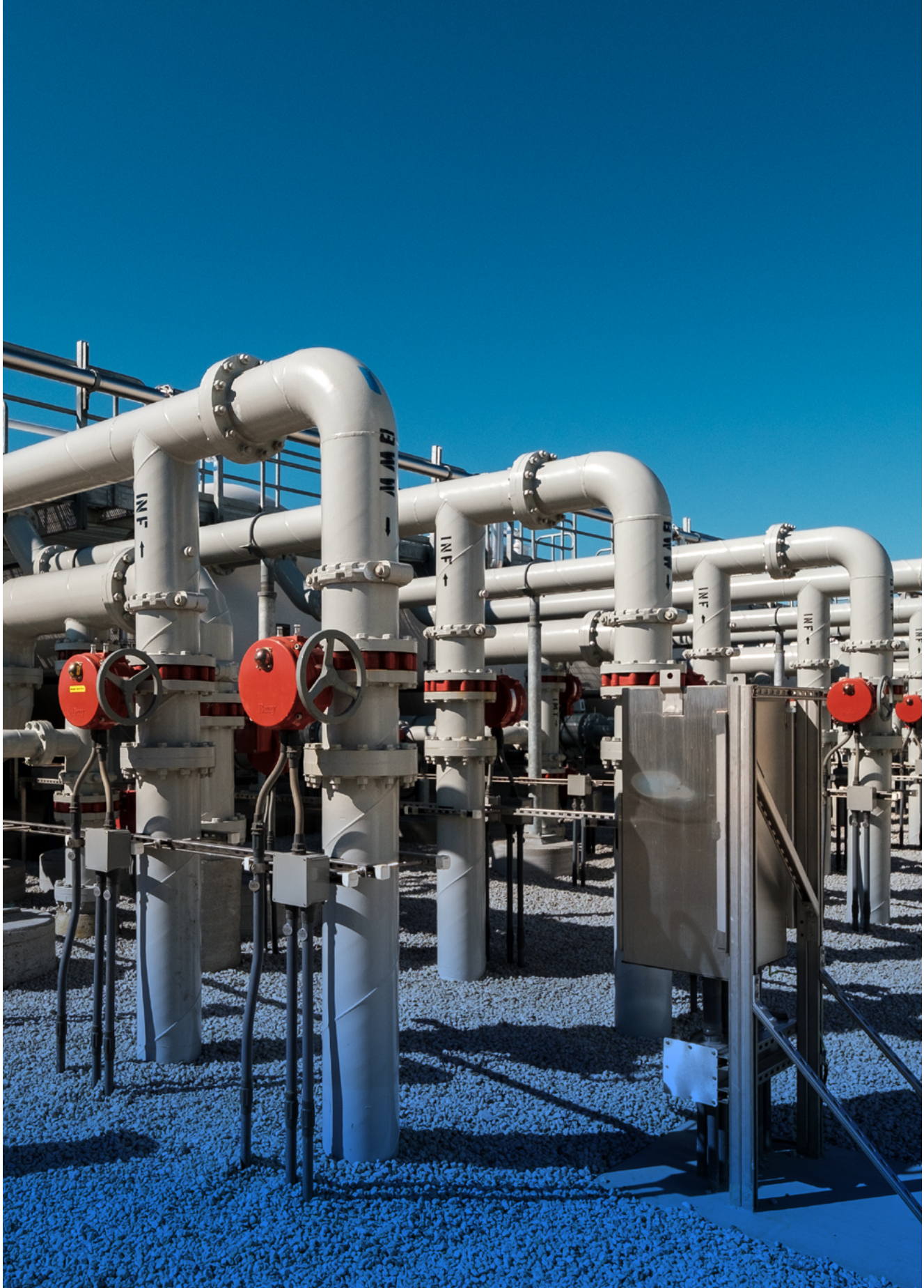
The Fallbrook Groundwater Desalter Project received LRP funding and produces 3,100 acre-feet/year of treated groundwater with a newly constructed groundwater treatment plant, pipeline and upgrades to a pumping station.
