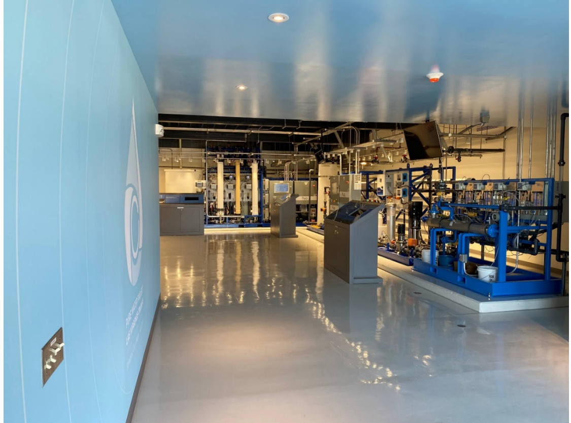
Figure 2 Interior of LVMWD Pure Water Demonstration Facility.
