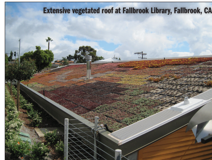
The extensive vegetated roof on this public library features modular units containing lightweight media and various drought-tolerant vegetation.
