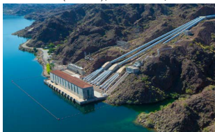
Whitsett Intake Pumping Plant
