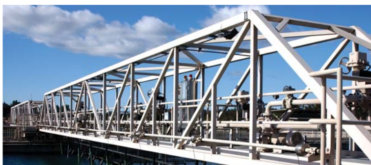
JENSEN WATER TREATMENT PLANT IN GRANADA HILLS
