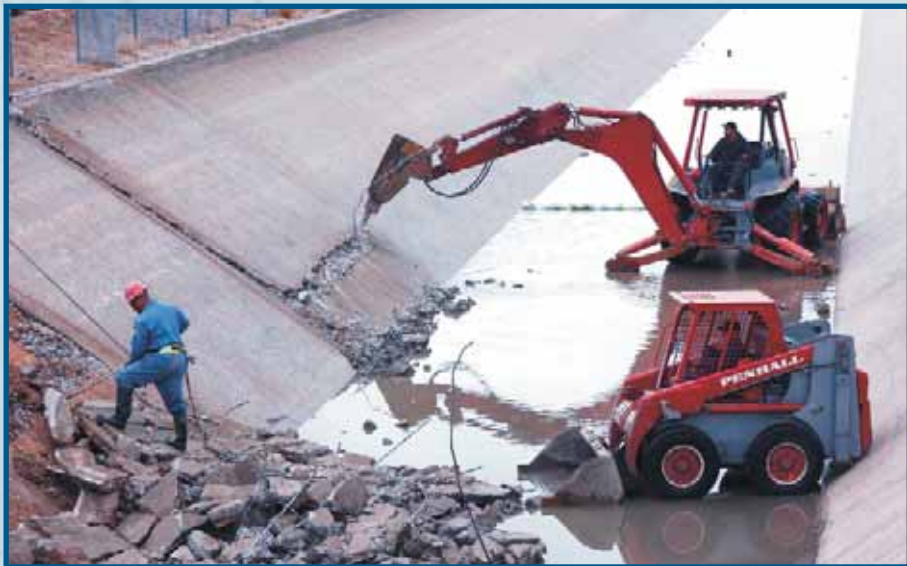
Metropolitan recently completed significant repairs to the Colorado River Aqueduct in order to maintain its conveyance reliability.
