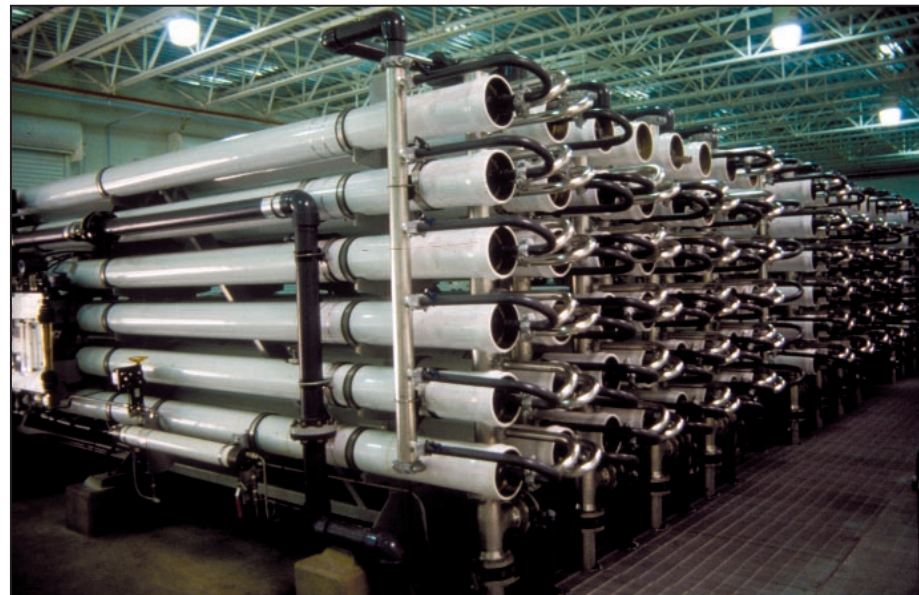
Desalting equipment used for groundwater recovery projects receiving funding from Metropolitan.
