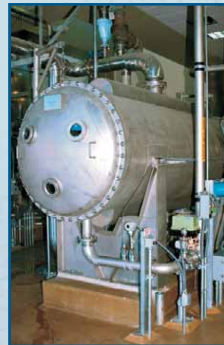
Ozone treatment is planned for all five of Metropolitan's water treatment plants.
