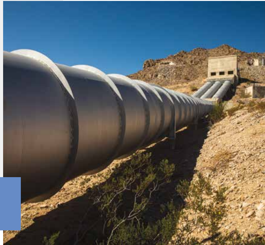
Photo: Iron Mountain Pumping Plant
