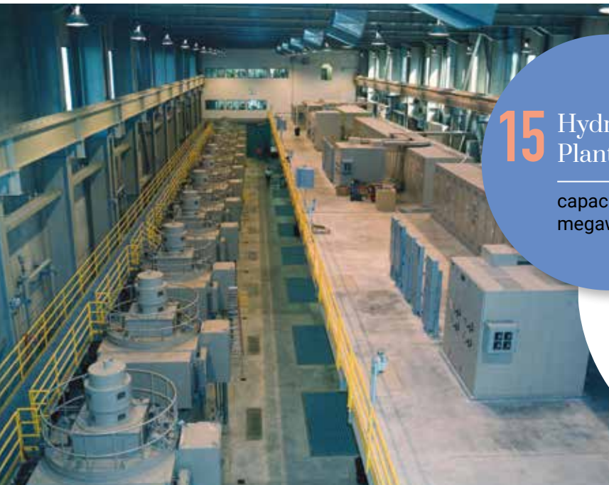
Photo: Wadsworth Pumping/Hydro-generating Facility
