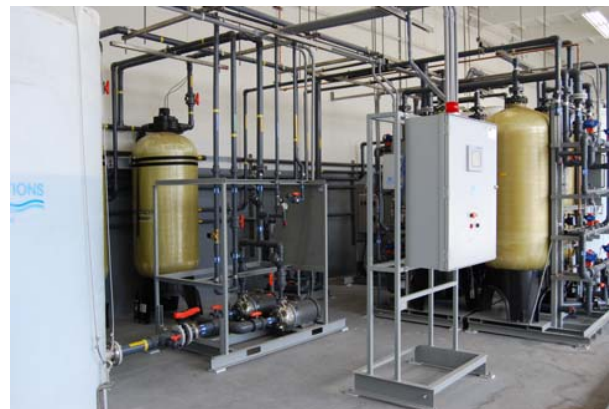
Marcel Electronics' Pump Skid Controller, De-ionized Water Recycling System
