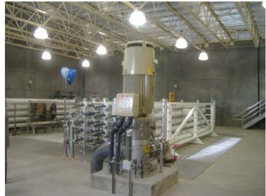
IRWD's Desalter Facility
